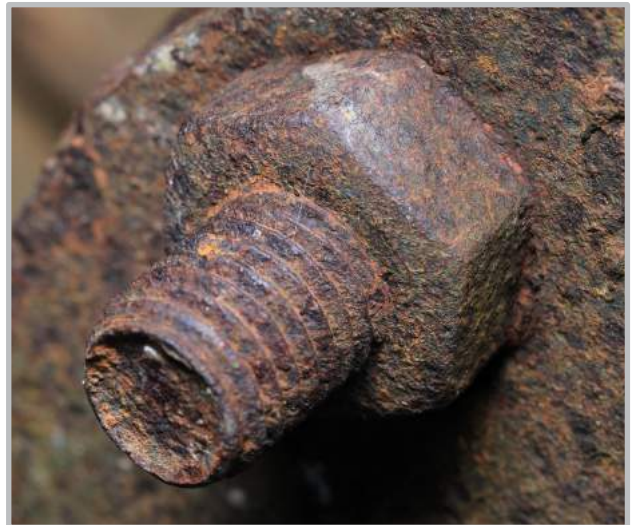
Corrosion of a nut and bolt
